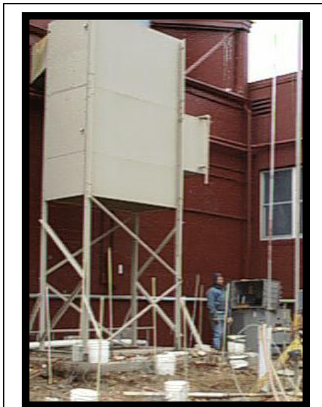
This air-handler, which was constructed on a 4-inch thick concrete pad, was elevated by fractures created at a depth of seven feet. Hydraulic fractures were created from a boring located at the lower, rightmost corner of this photograph – at the base of the yellow hoist unit. The staffs were used to measure uplift while the buckets protected tiltmeters.
